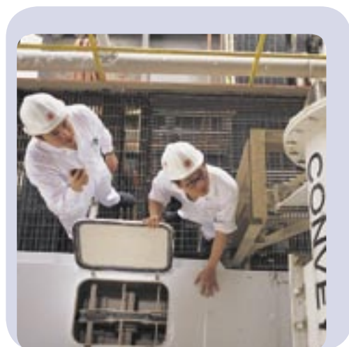
Our FGD plants can remove more than 90% of SO 2 in flue gas.
